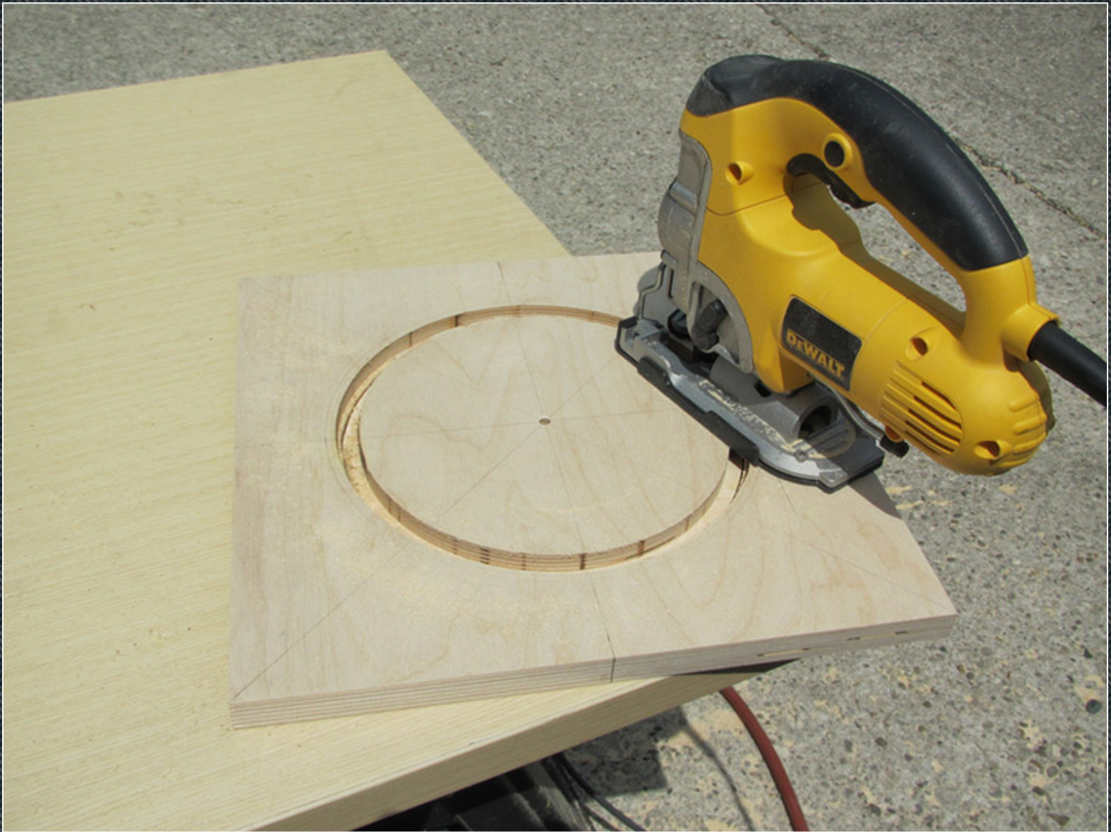
I finish cutting out the circle with a jig saw, leaving a ridge that will be routed off using the trim router.
